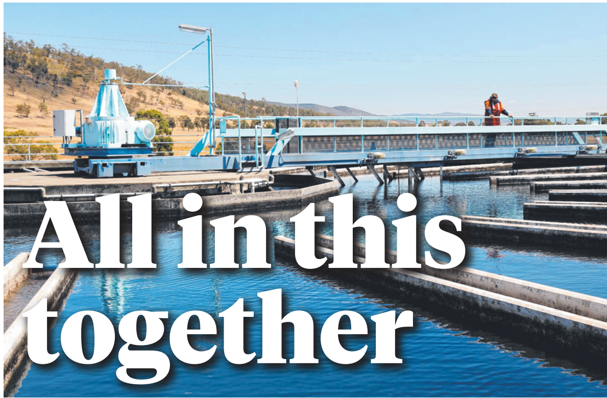
MAJOR FOCUS: A big upgrade is in the pipeline for TasWater's Bryn Estyn Water Treatment Plant near New Norfolk.
