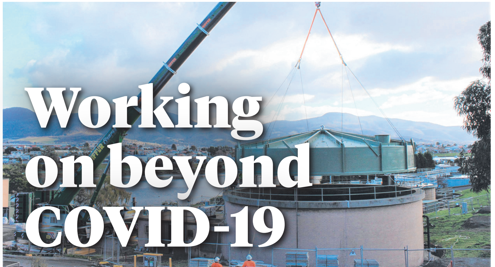
WORK GOES ON: Lifting a new roof on to the Prince of Wales Bay Sewage Treatment Plant digester tank as part of its $5.1 million upgrade.
