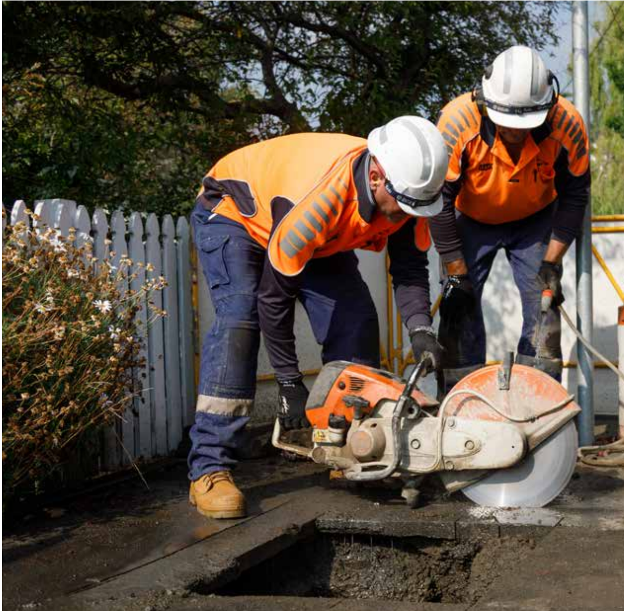
Darren Webster and Adam Tilyard cutting bitumen to access a leaking pipe in a residential area.
