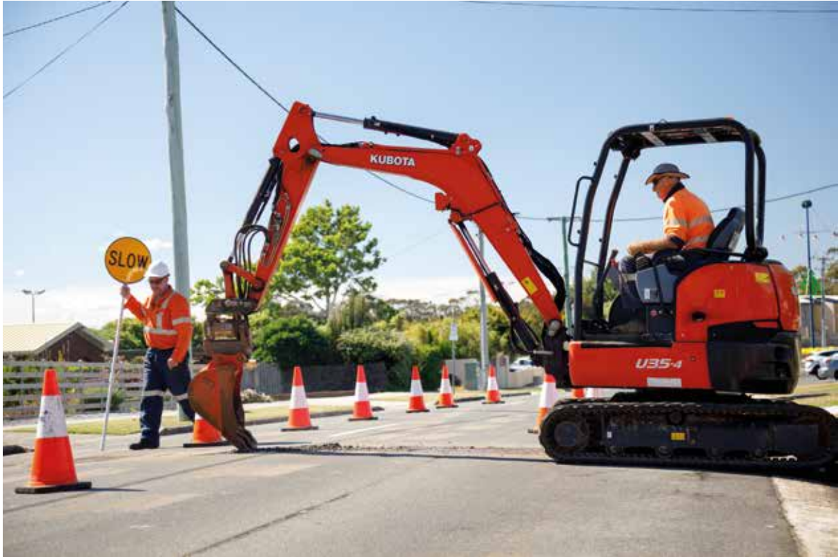
Works underway in Shearwater, northern Tasmania. TasWater's commitment to ensuring its assets are efficient and perform to national standards is an important strategic issue.
