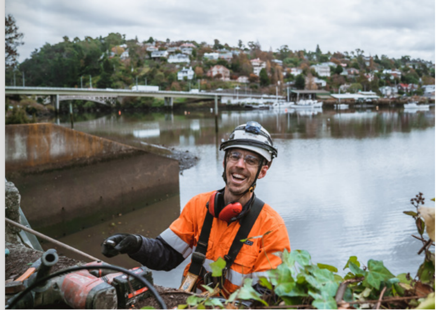
Project Manager, ADS Environmental Services, Manfred Faust installing flow gauges as part of the Tamar Estuary River Health Action Plan. Photo credit - Jade Higgs
