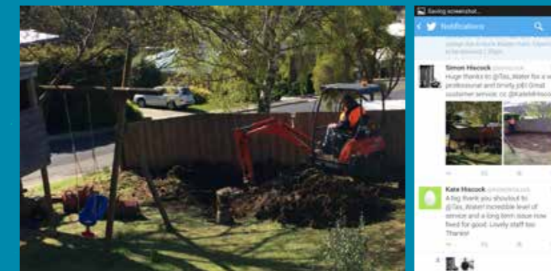
Left: The TasWater excavator at work digging up the Hiscock family's pipe. Right: The Hiscock family thank the TasWater team on Twitter.
