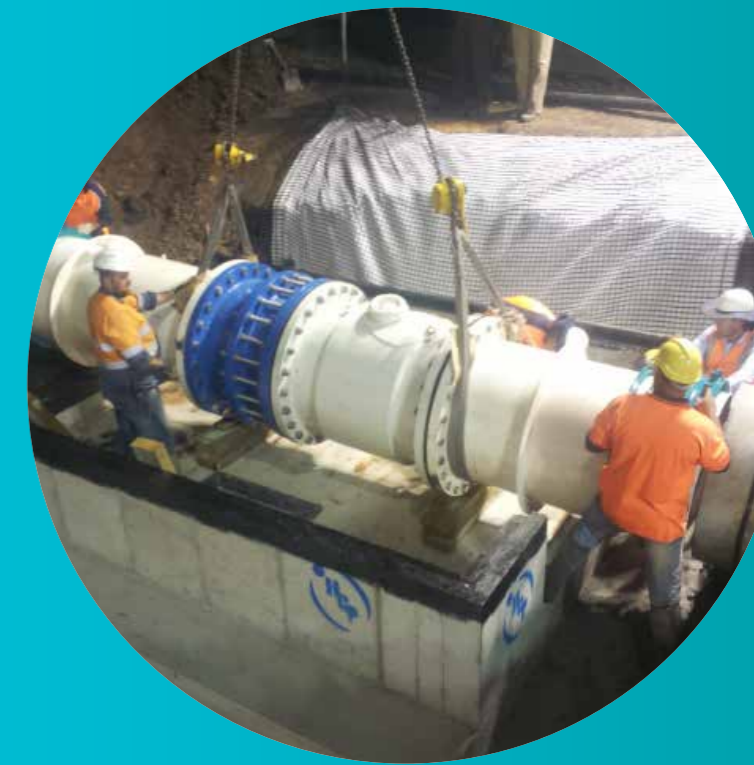
Crews hard at work on the 12 hour Installation project as part of the Ti Tree Bend STP upgrade.
