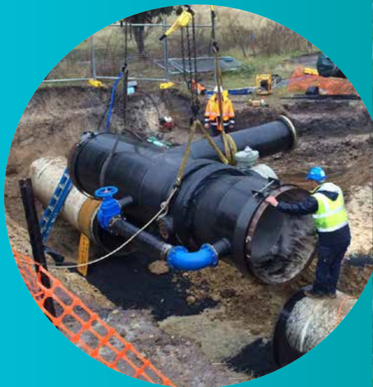
The team install the offtake to the West Derwent trunk main at Granton.
