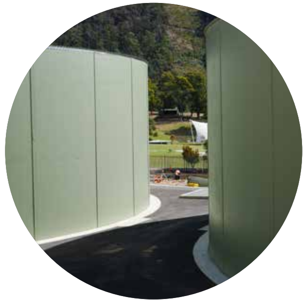
New water storage tanks at Tolosa Street, Glenorchy.
