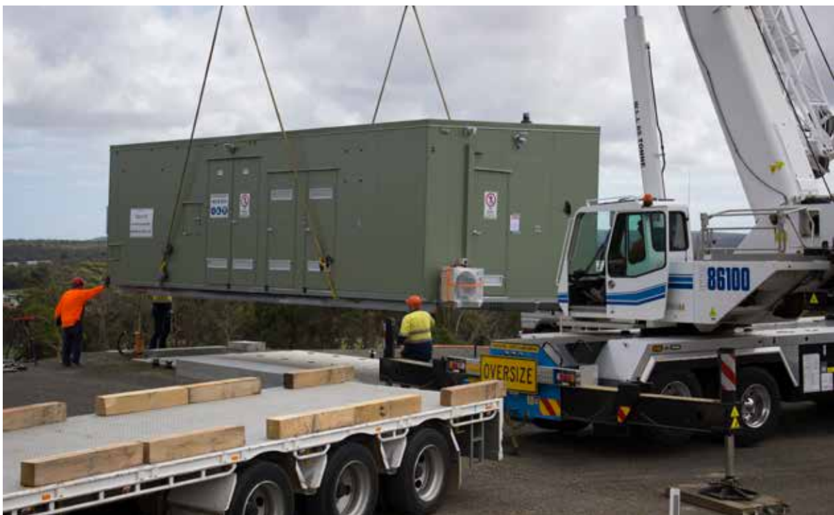
A prefabricated water treatment plant is lifted into place in Gladstone, part of 24glasses - RTWSP.
