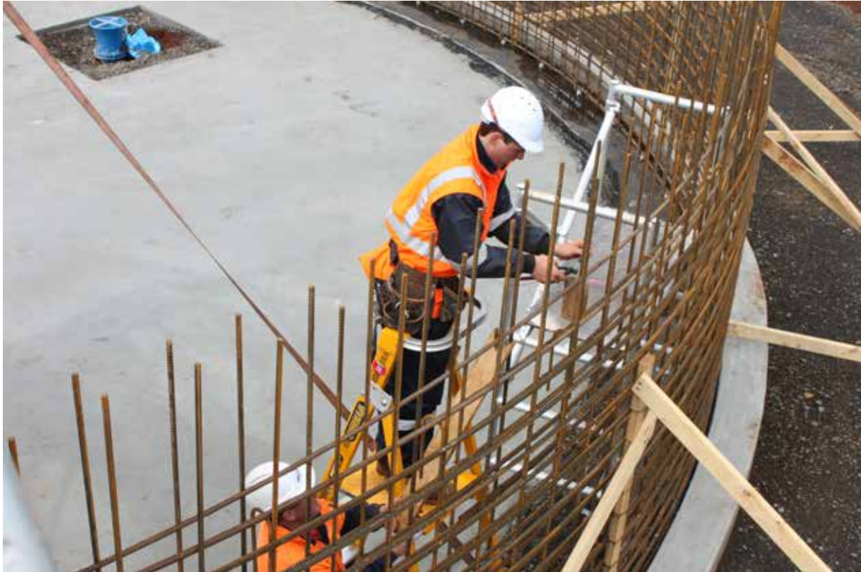
Building Ringarooma's new reservoir, as part of 24glasses - Regional Towns Water Supply Program.
