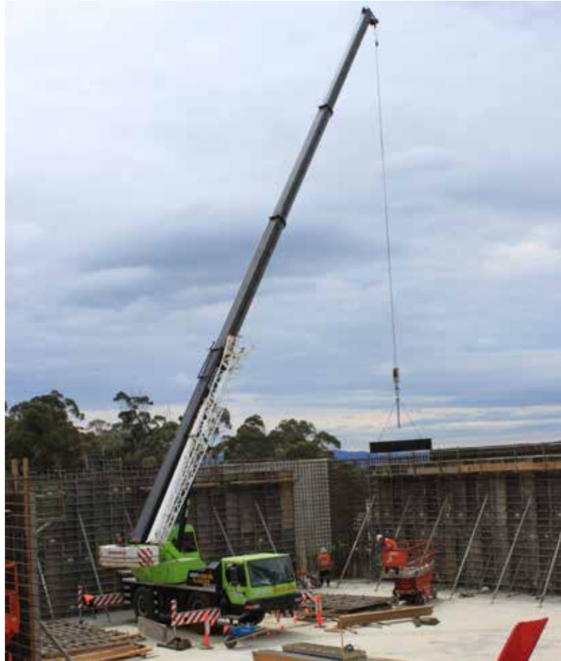
Construction of the Blackmans Bay STP, part of the broader Kingborough Sewage Upgrade Program.
