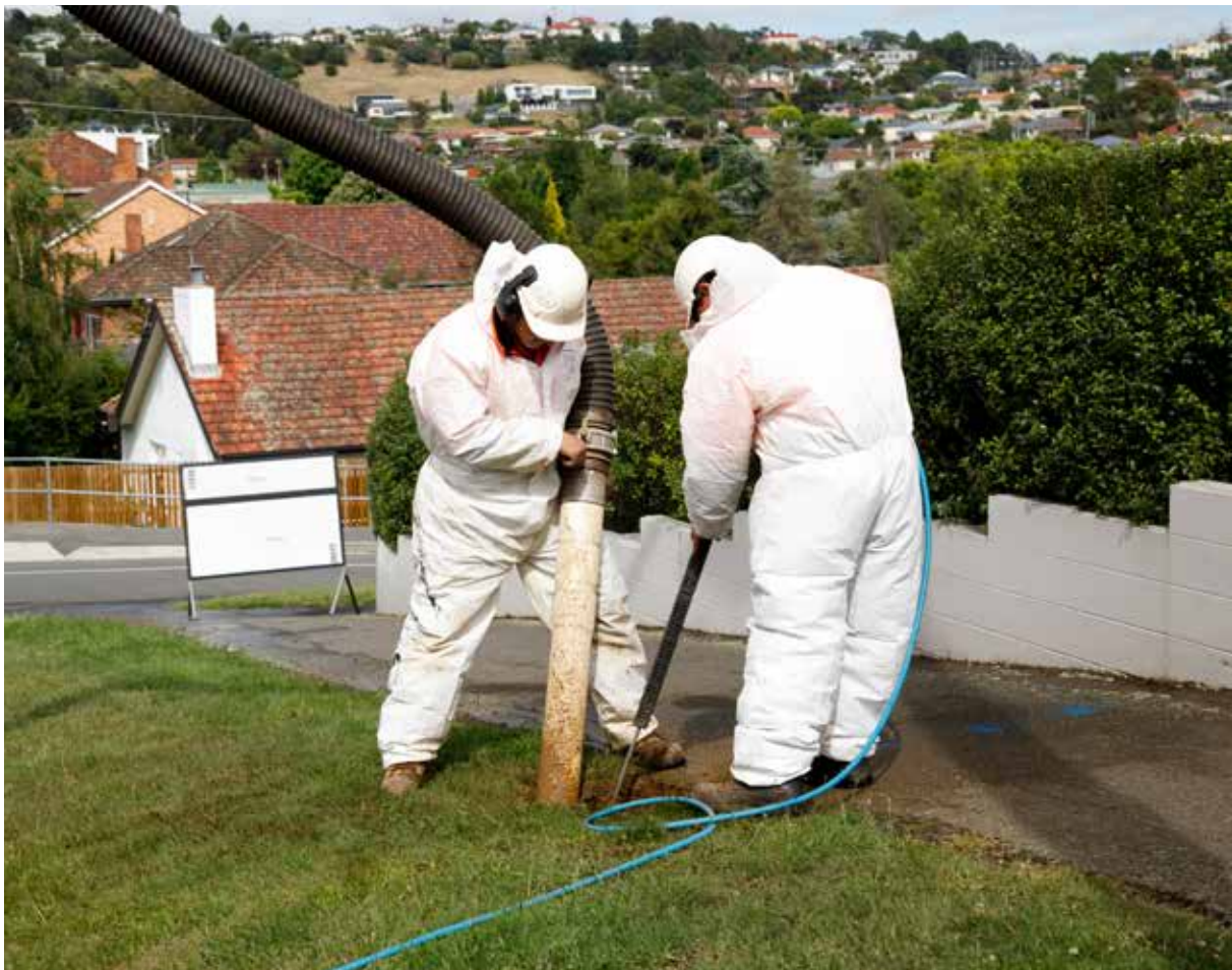
TasWater staff undertake sewerage maintenance works in Newstead in the state's north.
